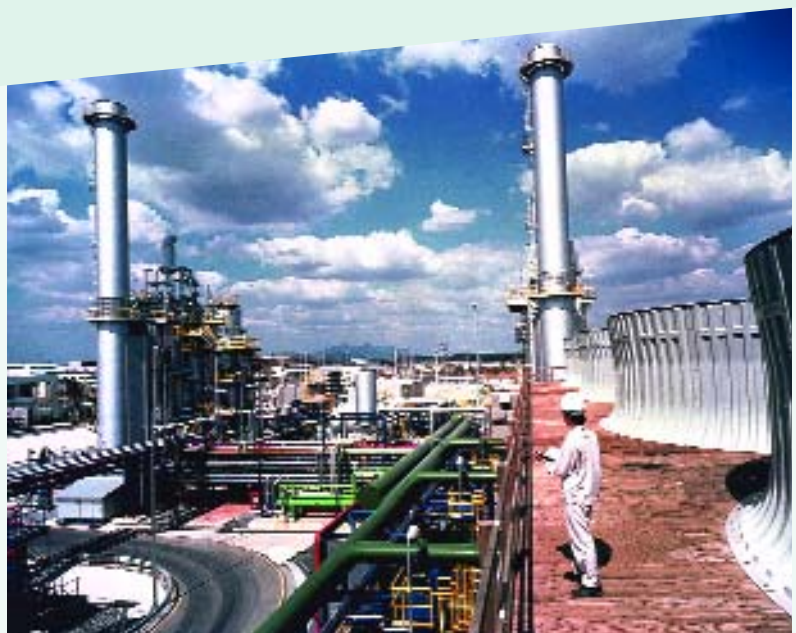
Above: Thai National Power (Pluak Daeng), Thailand
