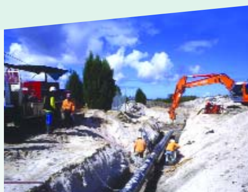
Above: SEA Gas pipeline, Australia
